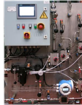
②Dosing unit and SCR control panel
