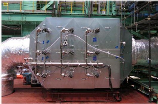
①SCR Reactor with Soot blower
